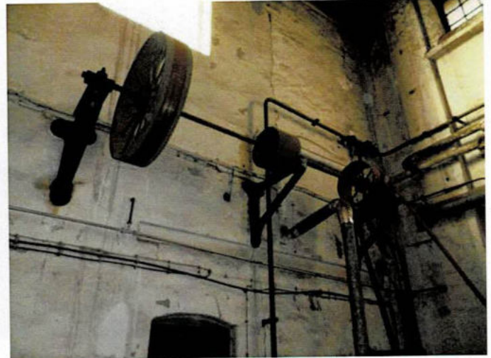
Transmission alter Dampfkessel
