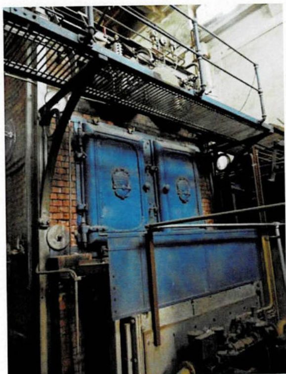
alter "Babcok" Dampfkessel
