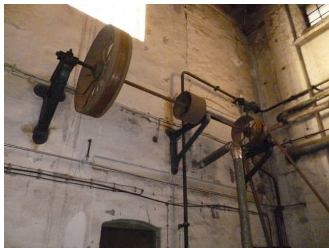
Transmission alter Dampfkessel (6)
